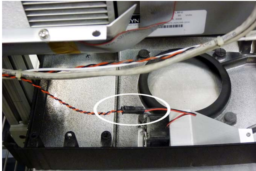
Figure 7 Fan power connector location
